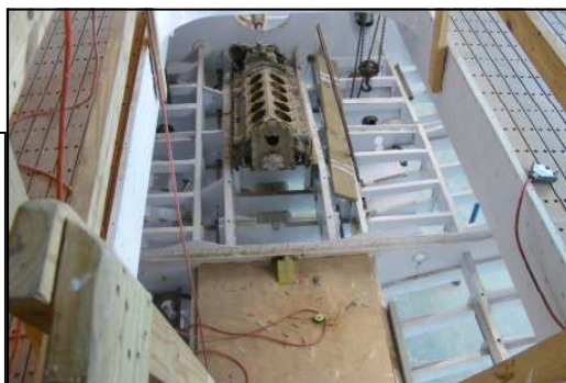
An engine block in the center engine position a temporary placement for alignment of shaft/framing.
